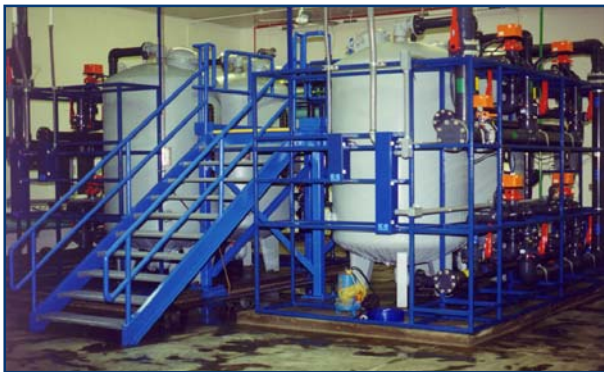
A 1.1 million GPD filtration system, Southwest Harbor, Maine
